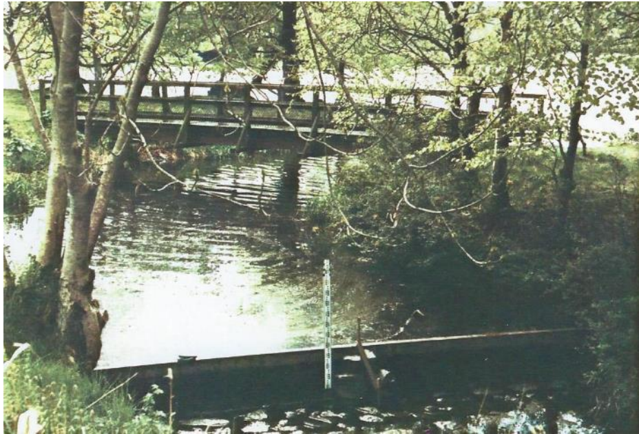
NORTH EAST OUTFALL, SHOWING STOP LOG SYSTEM. 1986.
